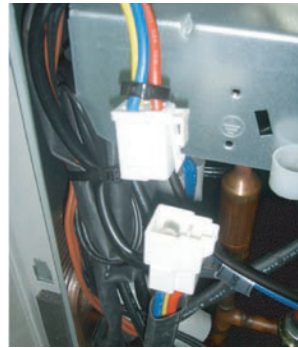
Compressor Wire Connection
