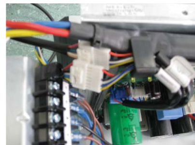
<fan motor middle connection>
