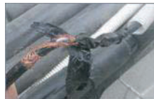
Cases of field defects
